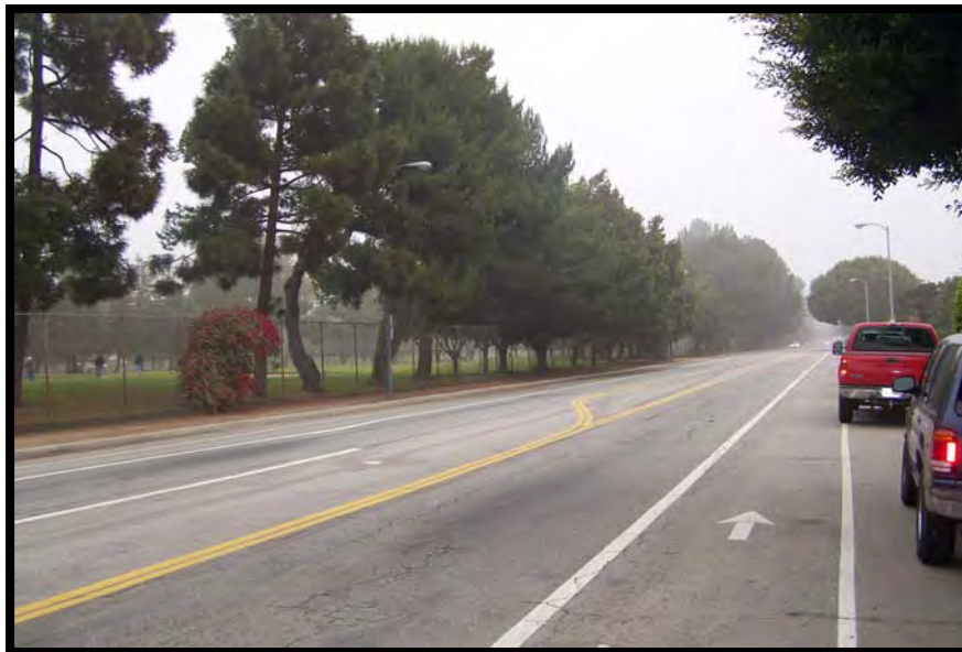
Photo A4. View to east-northeast from south side of Rose Avenue at Frederick Street, along proposed trench for force main (3) conduits in north half of Rose Avenue. Penmar Municipal Golf Course in background (Penmar Project Area).
