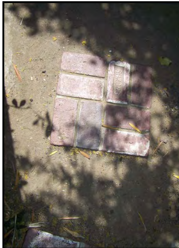
Photo A31. Simon brick paver footpath between Rialto Court and Crescent place (Rialto Court/Crescent Place Project Area).
