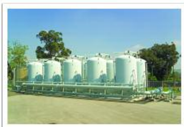
GAC vessels at Central Basin's Water Quality Protection Project.
